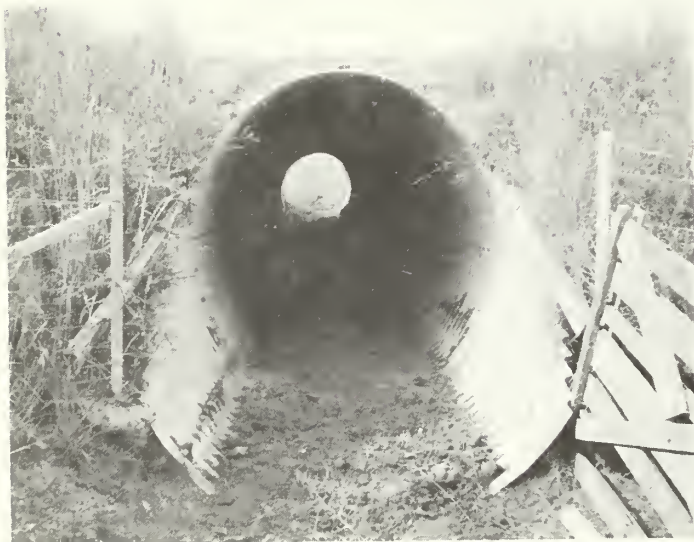
NORTH ENTRANCE: Notice pipe is mis- shapen
